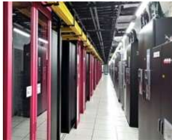
Fig. 2: AHFs at the server room in the second floor
