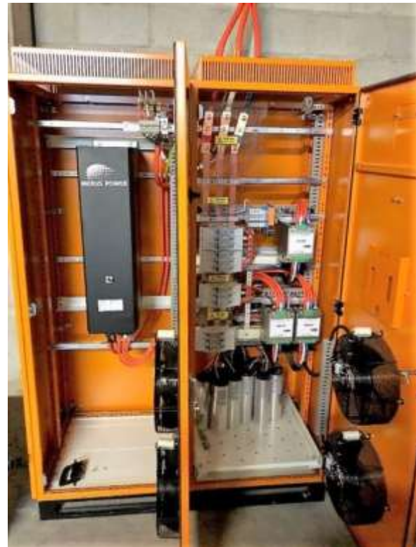
Fig. 3: HVC 415 V 50 Hz -72/+222 kvar located at feeder four
