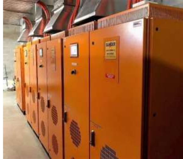
Fig. 2: Four HVCs at switchboard room
